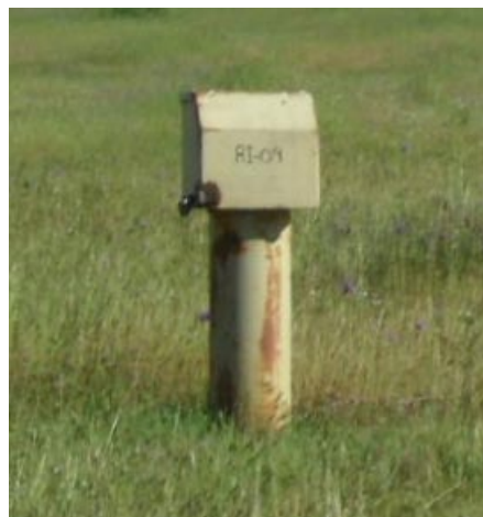
Figure 5: Sample wellhead completion (Photo)
