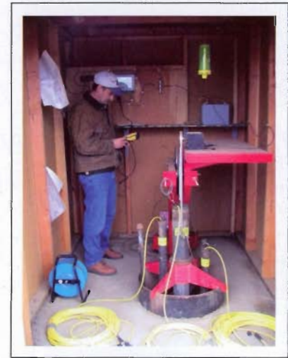
Figure 4. Above-ground portion of a cable extensometer with recording equipment.
